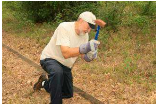
COT member Jerry Krampota installing galvanized edging strips on the Bayou Loop Trail.
