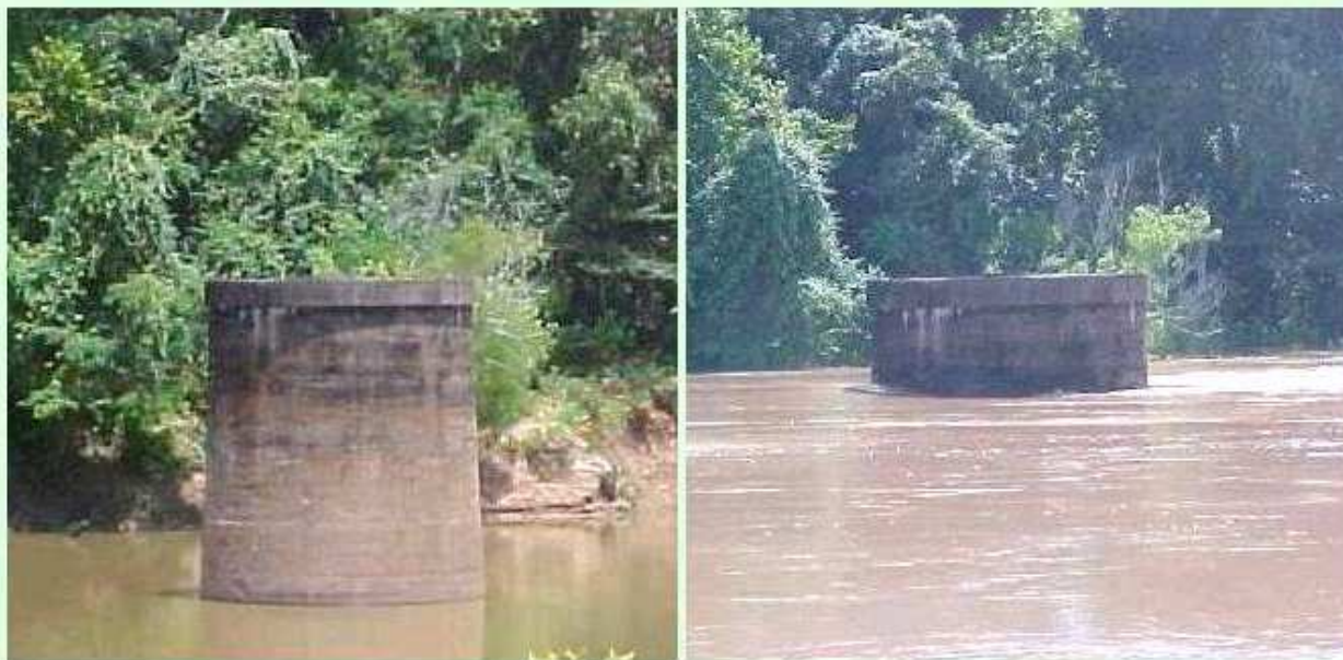
Pier from the west bank of the river, at low and high water Photos: Neal McLain
